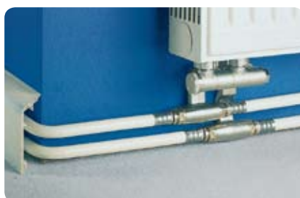
Fig 11. Radiator connection Courtesy of Hewing
