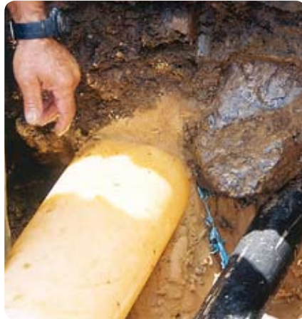
Fig. 24 Gas and water pipes with rock impingement, PE-Xa Courtesy of Golan
