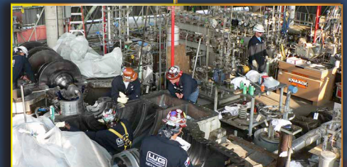
LyondellBasell employees and contractors working at the Clinton, Iowa facility completed a major maintenance turnaround operation in 2013.
